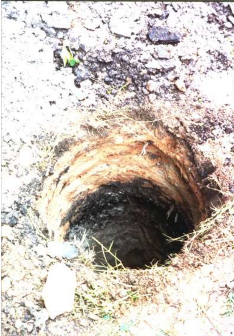
Fill material over wet soil
